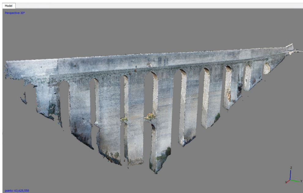
Fig. 2 Dense cloud of the North side of the Bridge of the Towers in Spoleto
