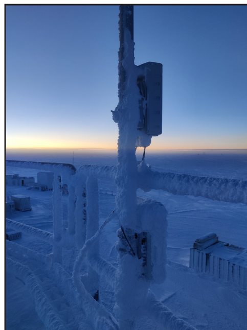
Fig. 10 Wi-Fi and mmWave antennas outside
